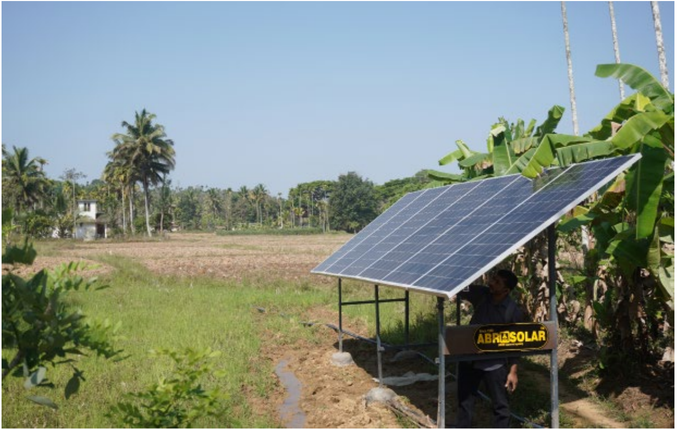
Solar Panels installed in Manivayal as part of the project
