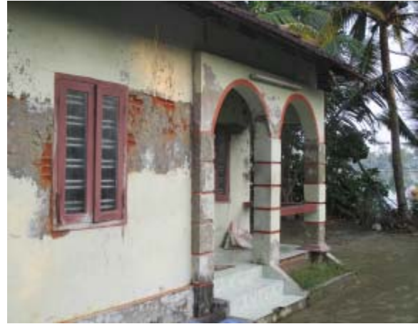
houses damaged by salinity
